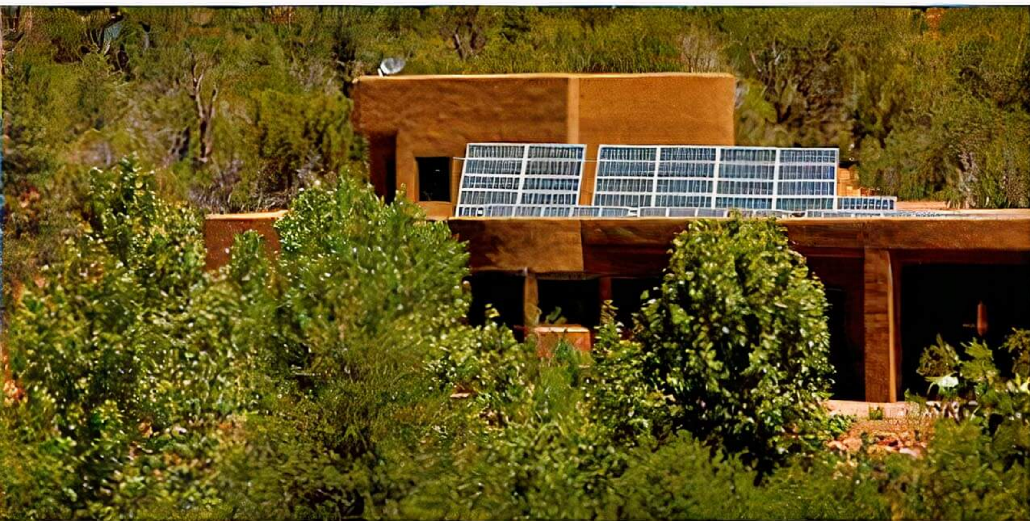
Solar panels collect heat for the Mohney home.
